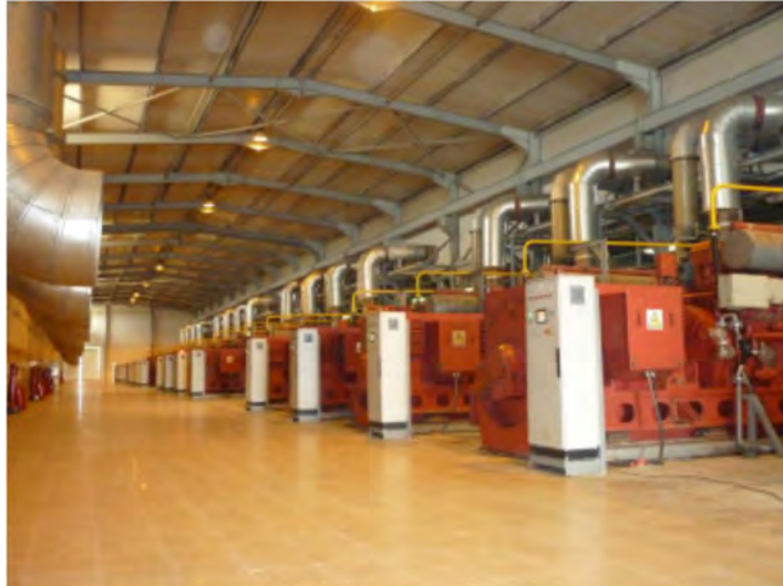
Figure VI.2.4 Cuba: distributed generation facility in Artemisa province
