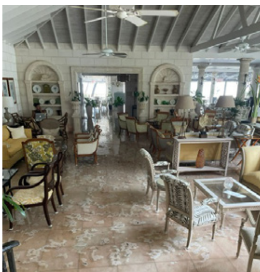
Image 6 Waterlogging damage: Coral Reef Club
