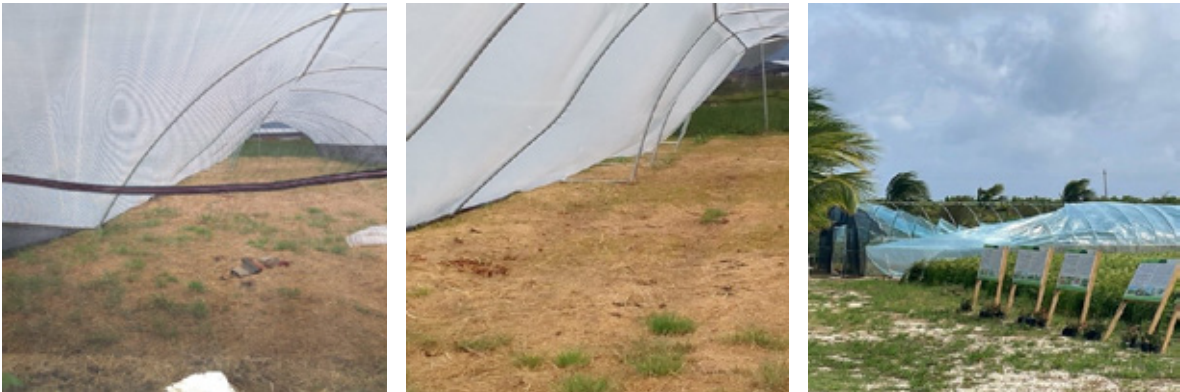
Image 4 Photographs of damages to public infrastructure in the agricultural sector
