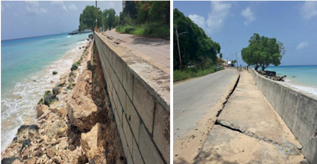
Image 10 Street Road inundated by storm waves
