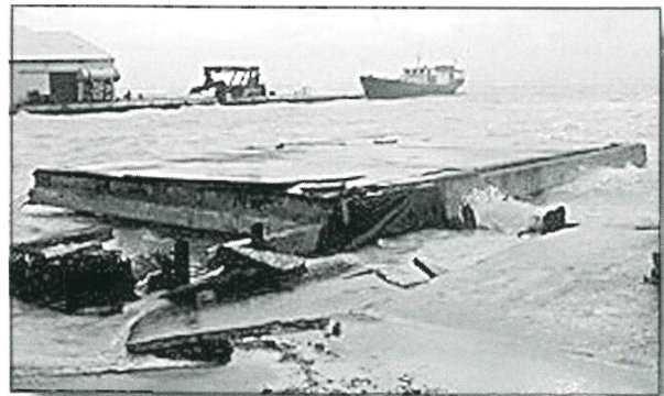
Remnants of a pier damaged by 1999's Hurricane Lenny. (Image: BBC World News Online.)
