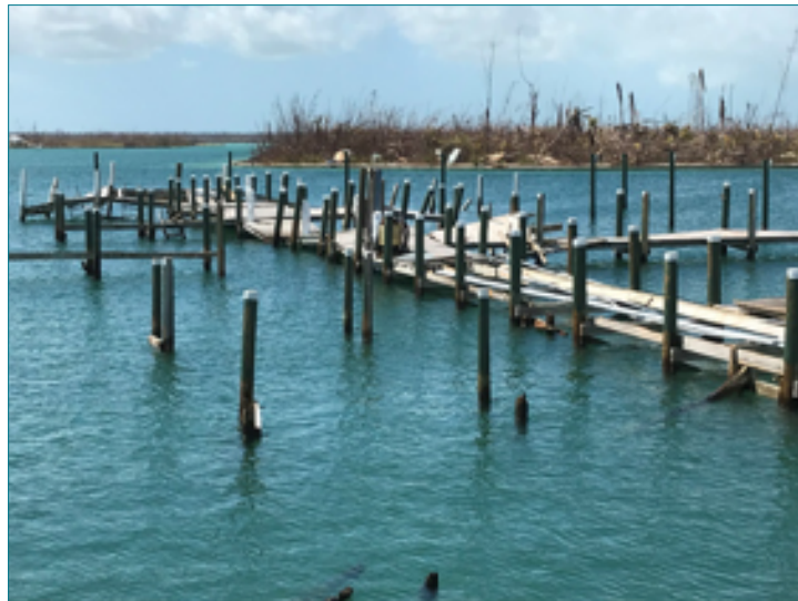
FIGURE 60. DAMAGED RECREATIONAL DOCK
