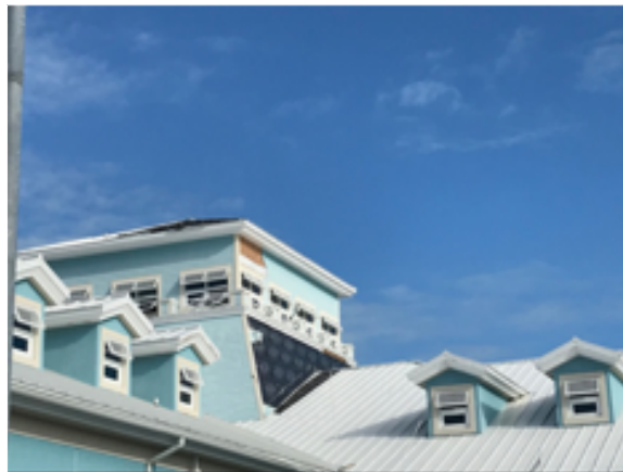
FIGURE 23. ROOF DAMAGE IN MARSH HARBOUR INTERNATIONAL AIRPORT
