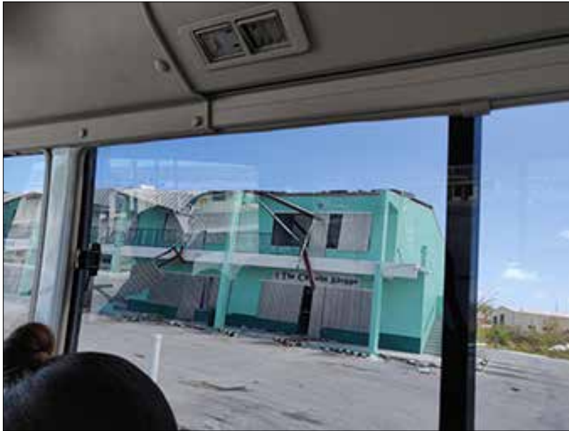
FIGURE 27. DAMAGE IN NON-STRUCTURAL ELEMENTS
