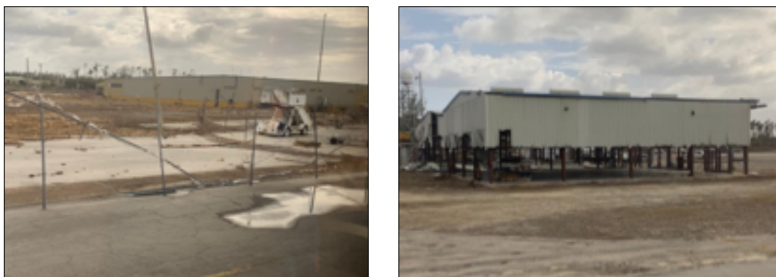
FIGURE 50. DAMAGE TO NON-STRUCTURAL ELEMENTS IN FREEPORT INTERNATIONAL AIRPORT
