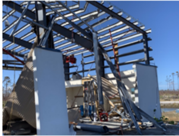
FIGURE 22. AIRPORT HANGARS DAMAGED IN MARSH HARBOUR
