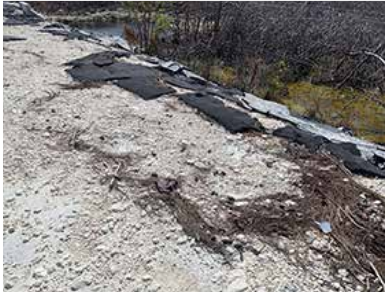
FIGURE 20. LACK OF TACK COAT AND NOT UNIFORM GRANULAR SUBBASE
