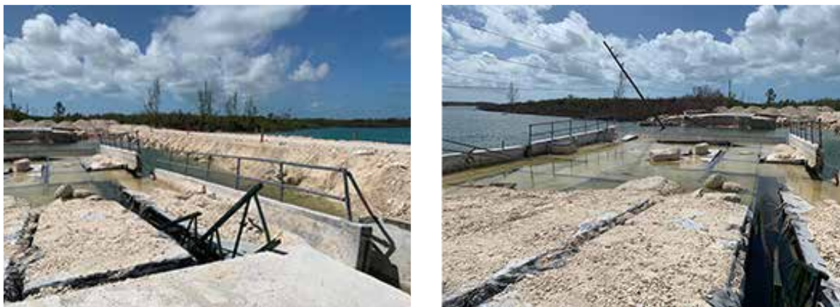
FIGURE 21. COLLAPSED BRIDGE IN NORTH ABACO
