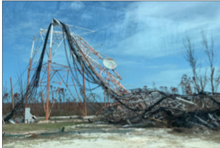
FIGURE 59. FALLEN CELLULAR TOWER, WITH DESTROYED BASE TRANSCIEVER STATION
