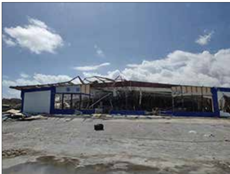
FIGURE 28. DAMAGE CAUSED BY WIND FORCE
