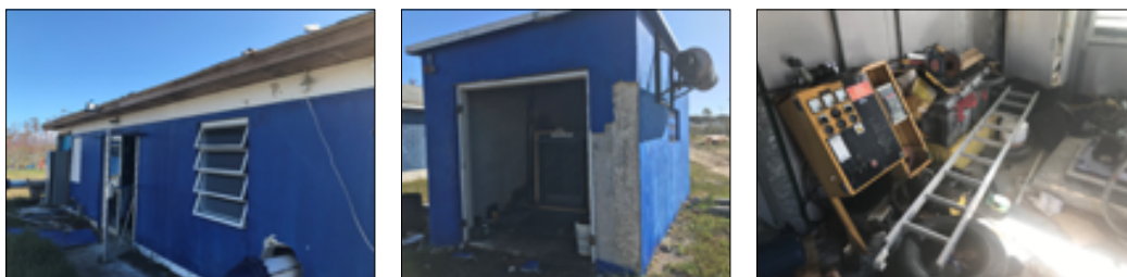
FIGURE 53. DAMAGE TO PUMP STATIONS IN MARSH HARBOUR AND TREASURE KEY
