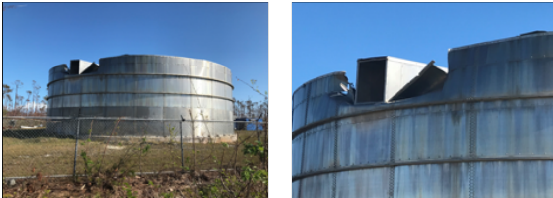
FIGURE 52. MAIN STORAGE TANK DAMAGE IN MARSH HARBOUR PUMP STATION
