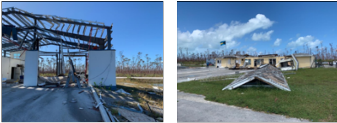
FIGURE 49. STRUCTURAL DAMAGE IN THE AIRPORT ON ABACO
