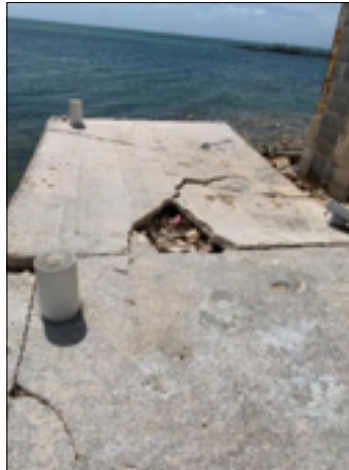
FIGURE 47. DAMAGED DOCK ON GRAND BAHAMA
