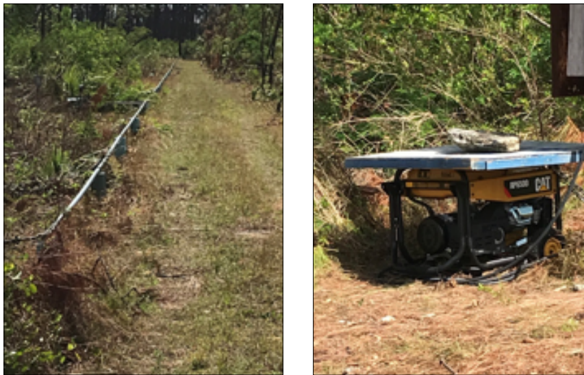
FIGURE 58. GROUND WATER COLLECTION SYSTEM / POWER BACK UP
