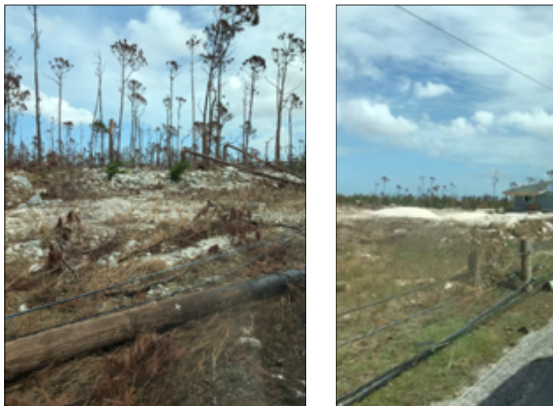
FIGURE 54. POWER DISTRIBUTION NETWORKS ON GRAND BAHAMA (VIA EAST END)
