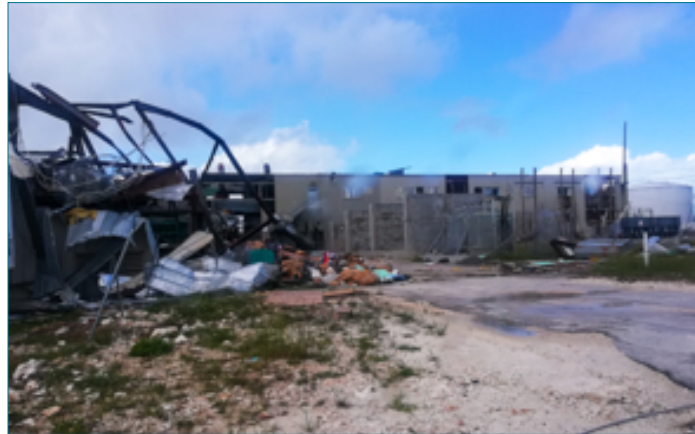
FIGURE 62. SEVERELY DAMAGED POWER PLANT AT MARSH HARBOUR
