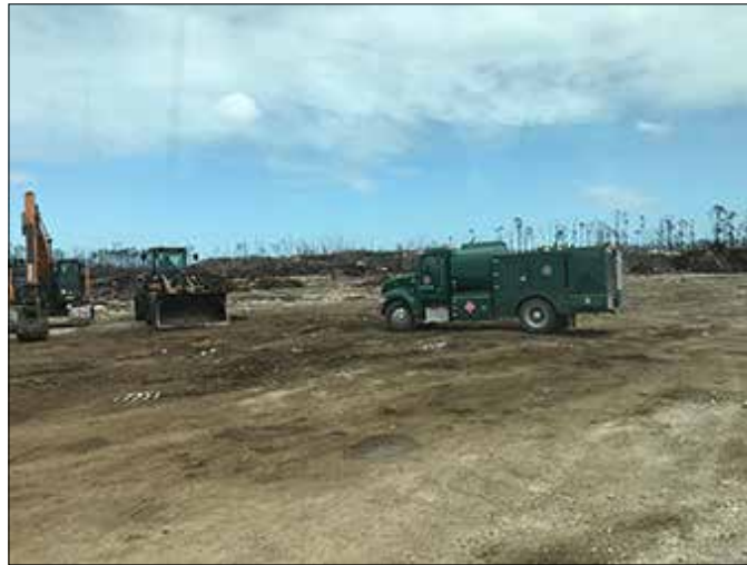
FIGURE 37. GRAND BAHAMA - OIL SPILL AT EQUINOR SOUTH RIDING OIL TERMINAL
