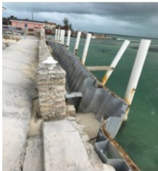
Image 4 - Damage on private dock facility at Bimini
