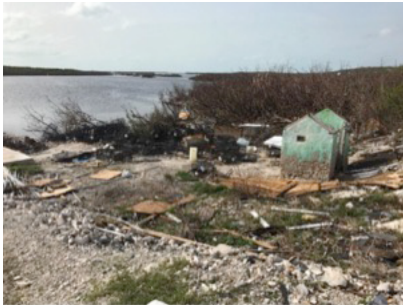
Image 12 - Ragged Island Fishing Dock Damage
