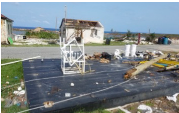
Image 15 - Damage in RO water plant- Ragged Island
