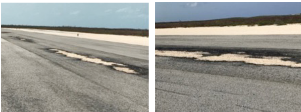
Image 9 - Damage in the Ragged Island Airport Runway
