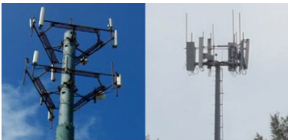
Image 16- Antennas connected to a tower at one point vs. antennas connected at two points using a bracing bar
