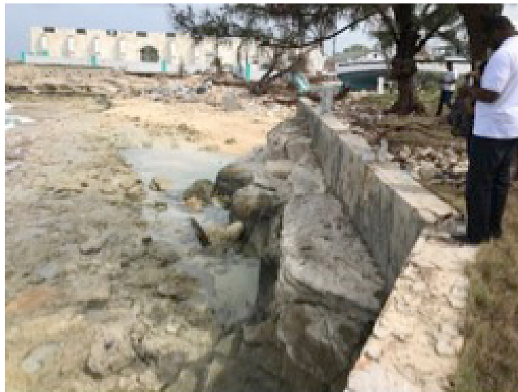
Image 8 - Seawall Damage Inspected in Great Inagua
