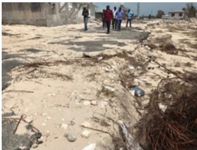
Image 7 - Damage in Roads at Salina Point, Acklins Island
