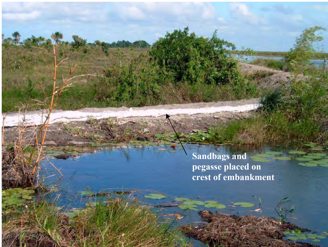
Photo 7 Embankment locations that were at risk from breaching
