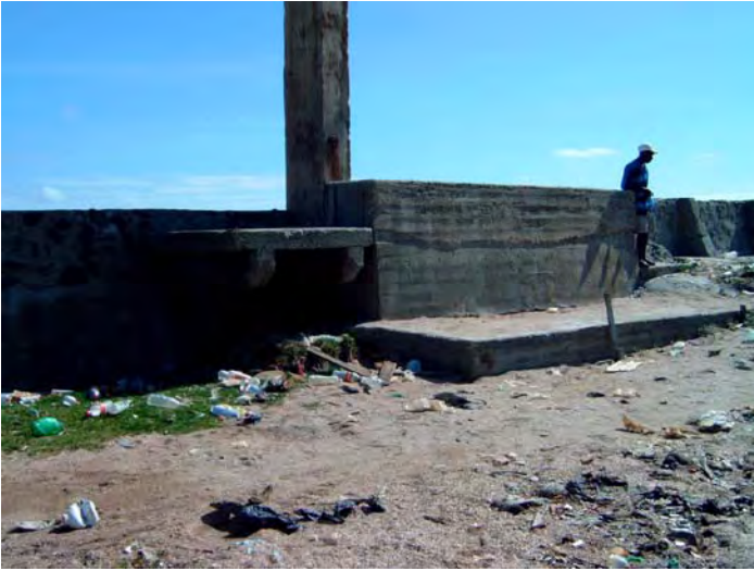
Photos 1 (above) and 2 (below) Derelict Koker and Resultant Ponding in Plaisance
