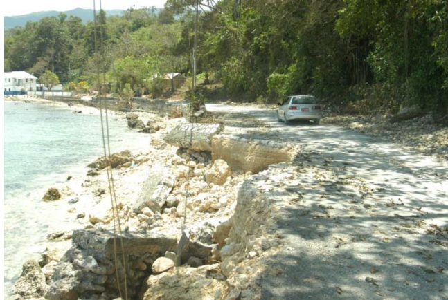
Environmental/Infrastructural damage, Hurricane Dean, Jamaica: June 2007
