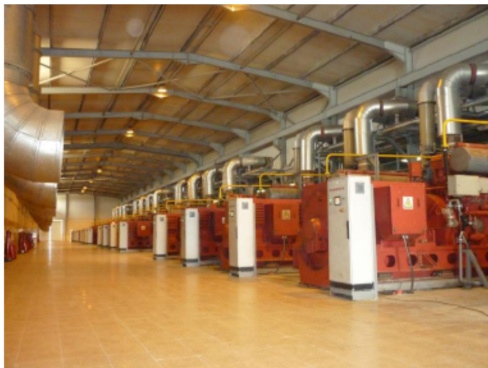
Figure VI.2.4 Cuba: distributed generation facility in Artemisa province
