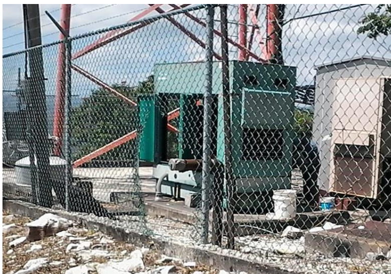
Figure 2 Vandalism damage to cellular site a
